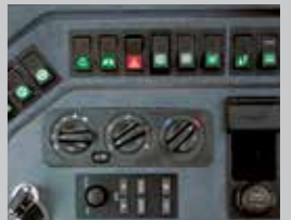
Instrument Switch Panel
