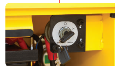
Master Switch A master switch disconnects the battery power to protect the electrical system from excess electrical drainage.
